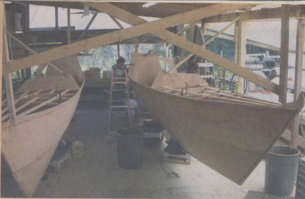
Both hulls were built side-by-side, braced to the shop floor and rafters to keep them aligned until they were rigid enough to be moved. Here you can see the forward deckbeams have been installed.
